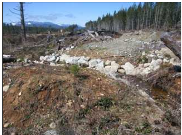
17. Culvert removed on deactivated road. Rip-rap remains in place to protect soil from erosion.
