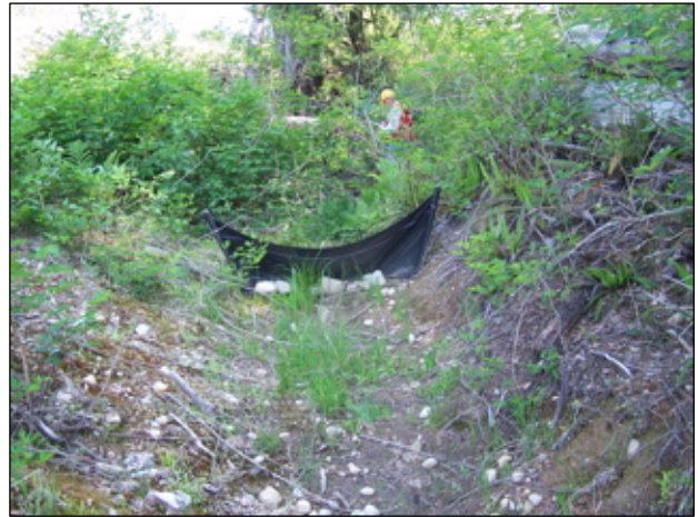
8. Silt fence installed on ditch before stream to help minimize sediment deposition.
