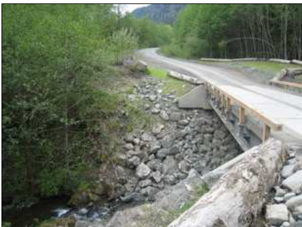
5. New steel girder, concrete deck bridge replaced an old log stringer, gravel deck bridge on this old, heavily used main line. Note use of rip-rap and grass seeding.
