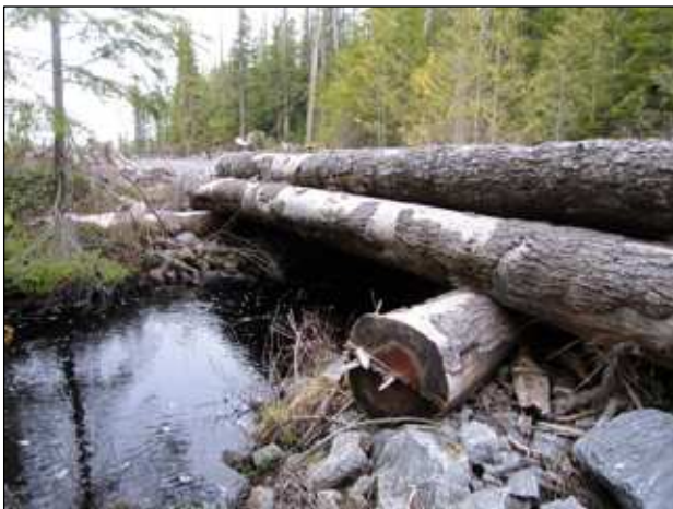
11. Large wood box culvert; sill logs well back to leave clear channel clear channel.
