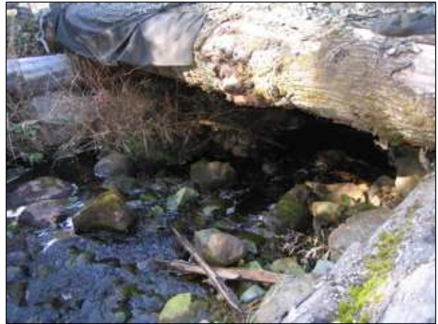
14. Wood culvert with sill logs well back leaving channel undisturbed. Note use of geo-fabric used to contain fines.
