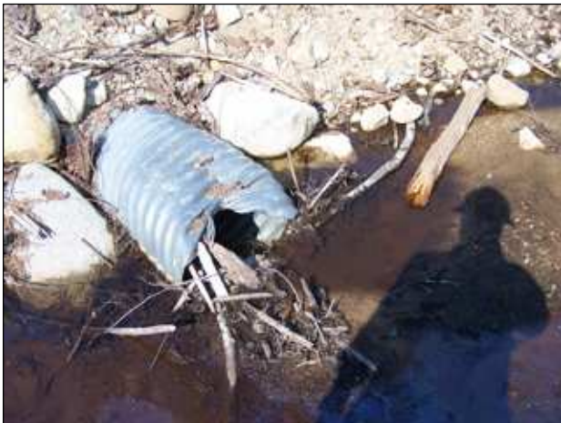
9. Culvert inlet partially blocked by sediment build-up. Digging a sediment trap would help here.
